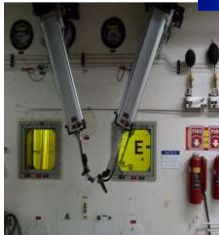
Remote Sizing in Dry Transfer Cubicle
