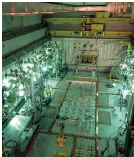
Hot Fuel Examination Facility, located at the Materials and Fuels Complex at DOE's INL Site in Idaho.
